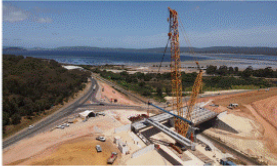
Albany Ring Road Project under construction 2023 * Image courtesy of Main Roads WA
