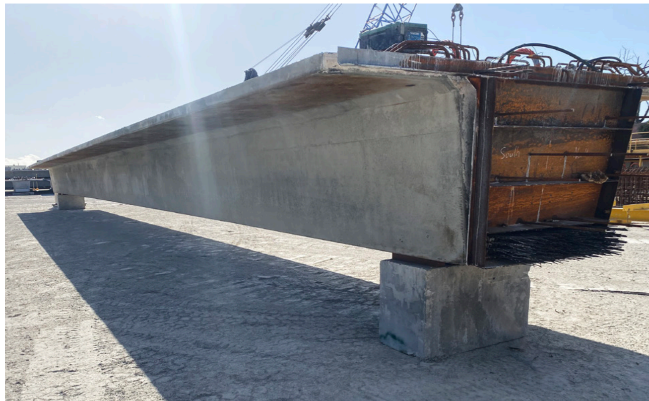
First beam cast in new multipurpose, high-capacity adjustable stressing bed – Bennett Brook Bridge
