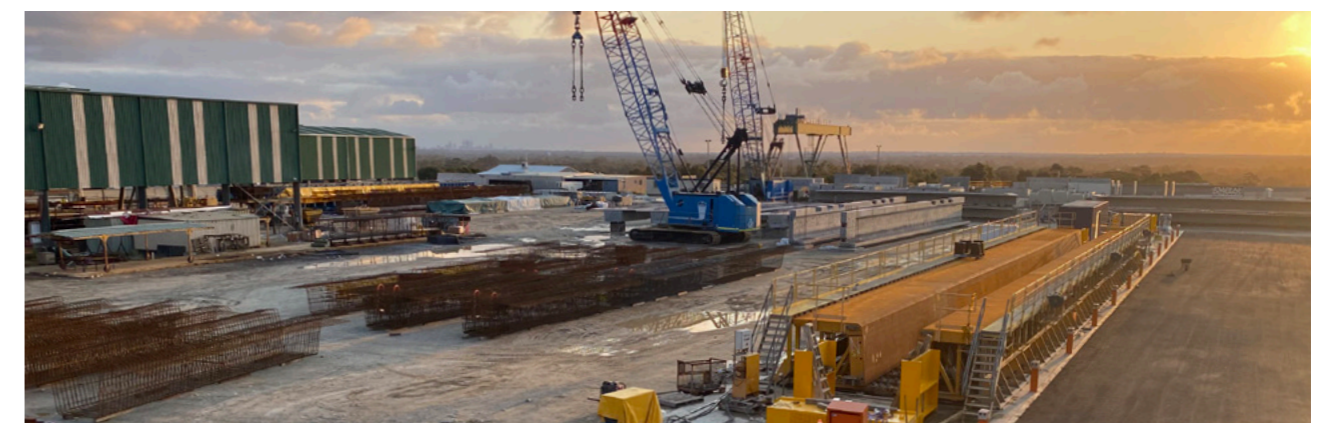
Above: New multipurpose, high-capacity adjustable stressing bed production facility Opposite: Bayswater Train Station Beams in the new storage area awaiting delivery
